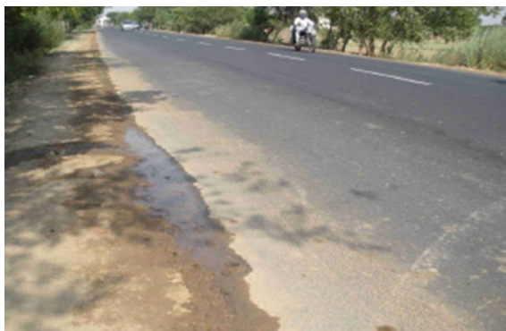
Fig. 7 Surface water ponding (nonconformance)
