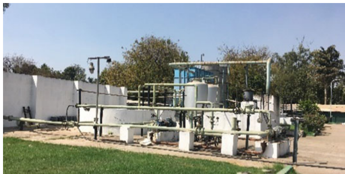
Fig. 1 IFFCO wastewater treatment plant
