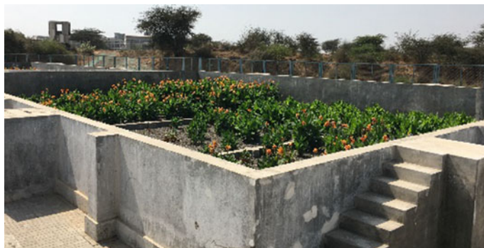
Fig. 4 DEWATS (plant gravel filter)
