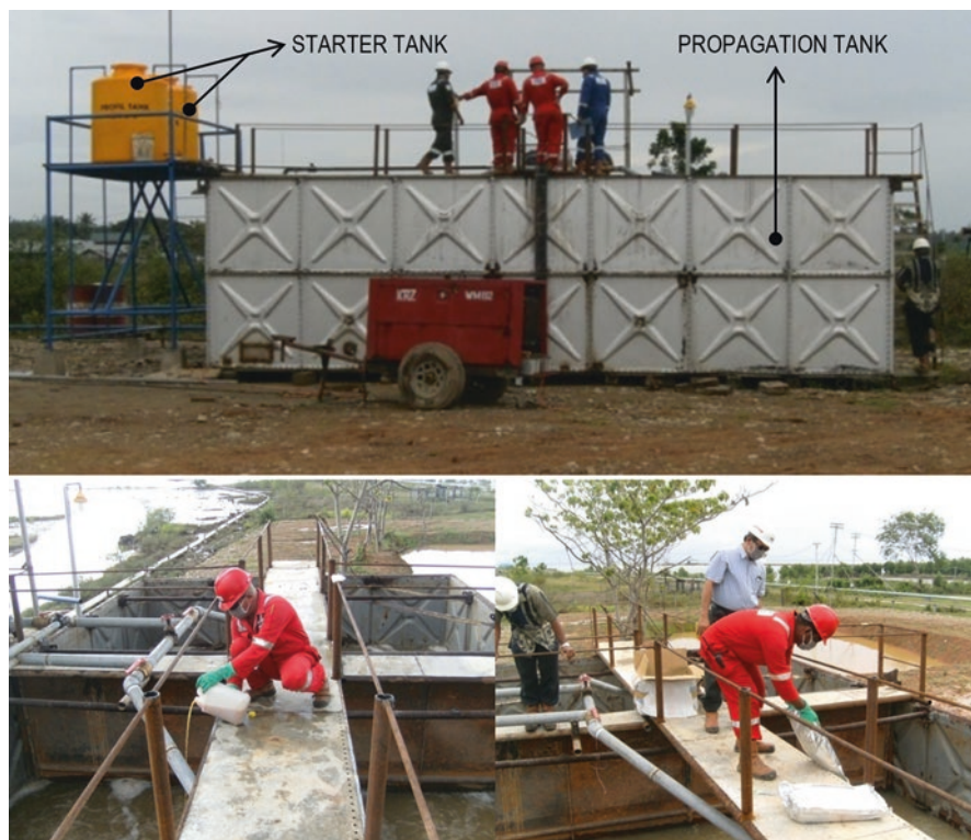
Fig. 7.12 On location production of petrofilic consortia and biosurfactants producing microbe on a 56 m 3 tank to enhanced the bioremediation process performance, (upper image) bioreactor installation, (lower image) nutrient and carbon source addition
