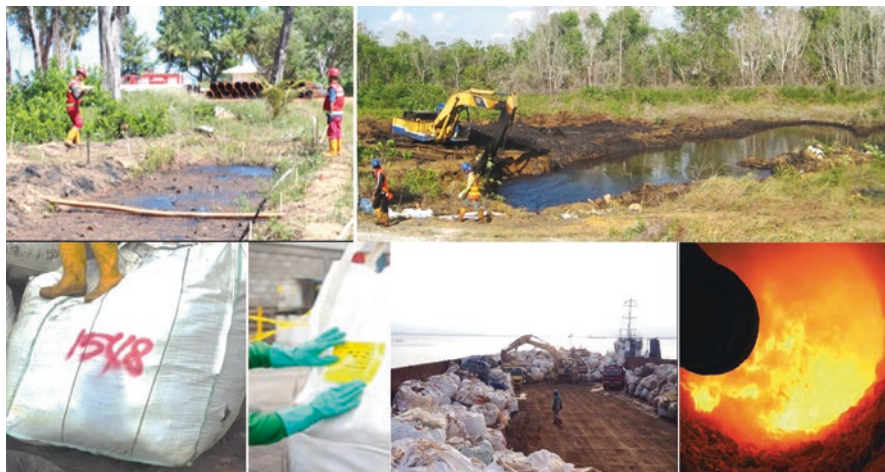
Fig. 7.5 Cleanup process of abandoned oily sludge pit (upper left to lower right): site investigation → excavation → containment → labeling → transportation → coprocessing in cement kiln
