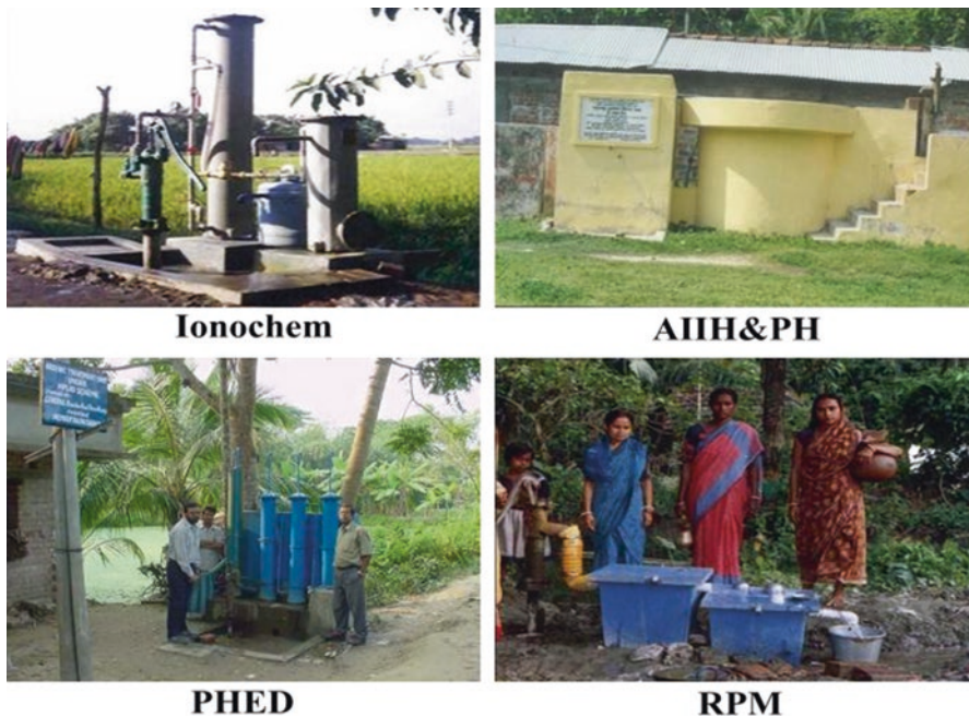
Fig. 3 Arsenic Treatment Units with hand pump operated tubewells
