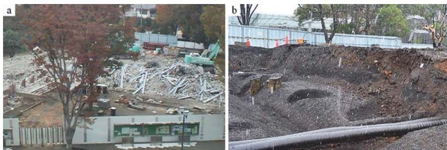
Fig. 1.16 Photo (a) shows the construction area where Andosols have been located in the research area. Sealants consisting of asphalt, concrete, and interlocking blocks were removed prior to the start of construction. Photo (b) shows the ground surface being prepared for new buildings. This site provided a valuable case to have a survey between demolition and reconstruction of buildings
