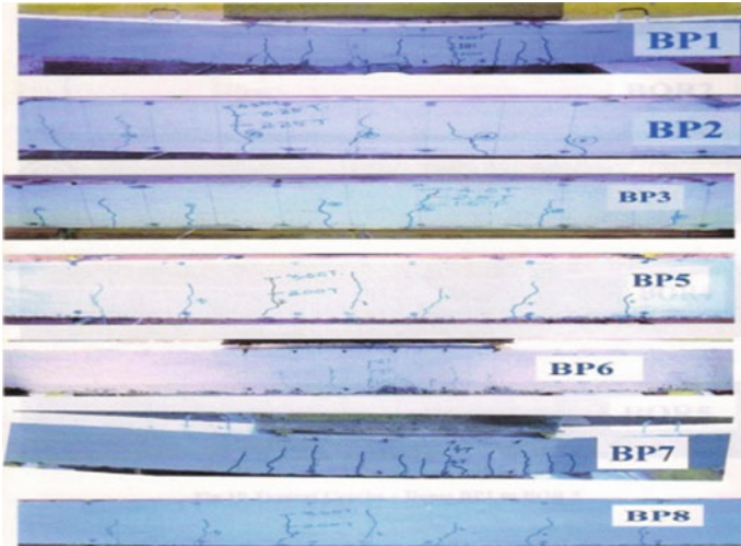
Fig. 4 Crack patterns in control beam
