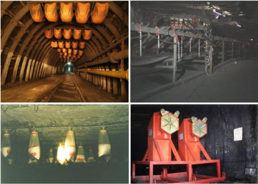
Fig. 5. Clockwise from top left to bottom right: water trough (China), active explosion barrier (South Africa), BatBag (South Africa and Australia NSW), active roadway barrier (China)
