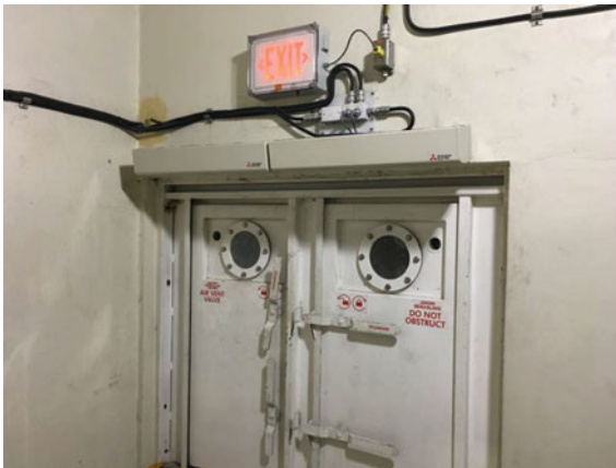
Fig. 3. Air curtain installation arrangement in a 250-person refuge chamber at the GBC mine
