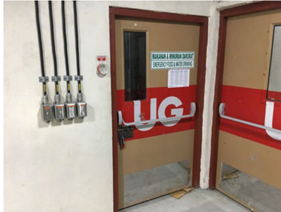
Fig. 8. Emergency food and drinking water storage room in a dual-purpose lunchroom/refuge chamber
