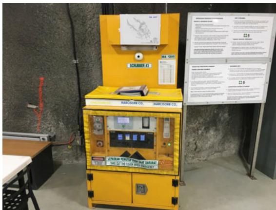
Fig. 7. Protective covers for life support equipment in a 250-person dual purpose lunch room/refuge chamber
