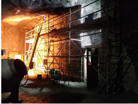
Fig. 11. Bulkhead under construction at a 500-person dual-purpose lunchroom/refuge in the GBC mine
