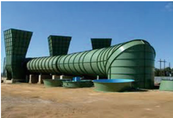
Fig. 2. Three exhausting fans in parallel with a well-designed bend to minimize shock loss
