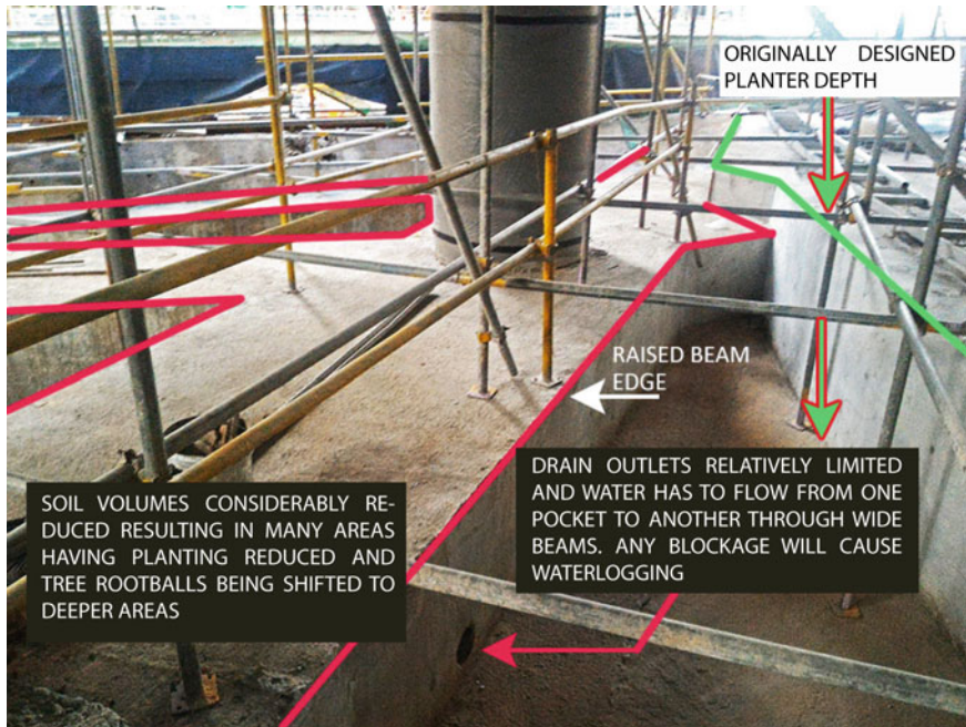
Fig. 11.2 Planter encroached by beams; Credit to ICN Design International
