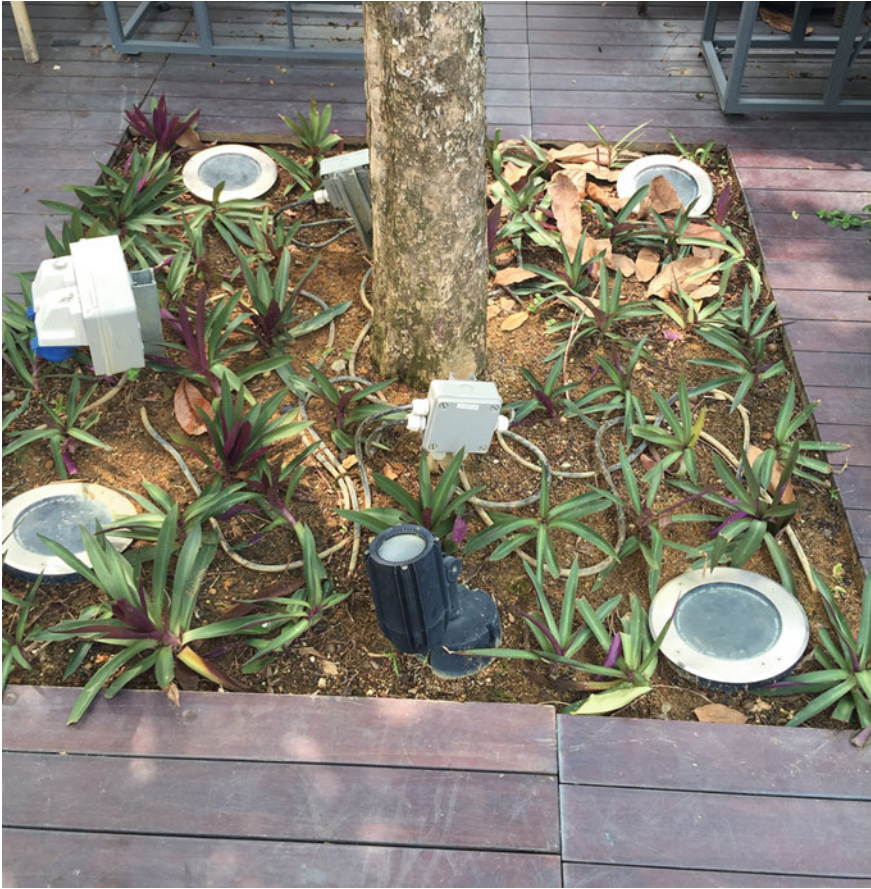
Fig. 11.3 Tree planter, big lights and junction boxes; Credit to ICN Design International
