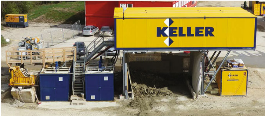
Fig. 14 Overview of Desander and Filterpress setup
