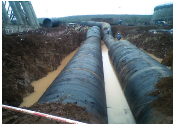
Fig. 6 Buried pipe experienced distress due to floatation
