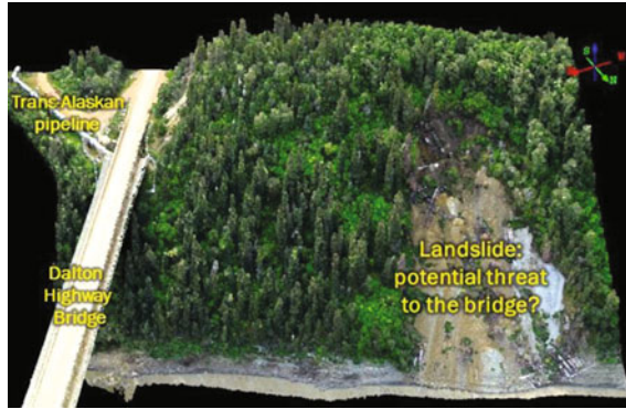
Fig. 3 Digital photogrammetric 3D point cloud of the Yukon River Bridge and nearby landslide in 2014
