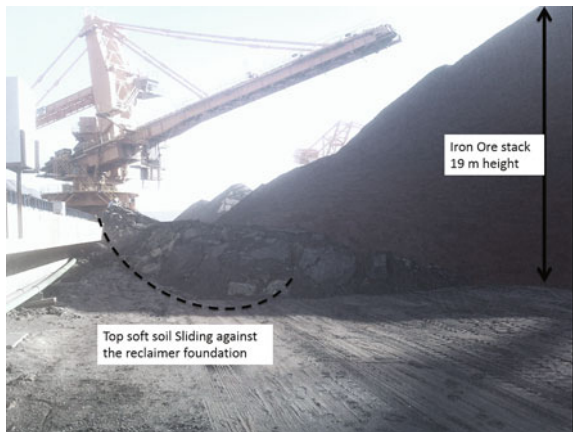
Fig. 9 Lateral sliding of soil due to rapid filling of iron ore stock
