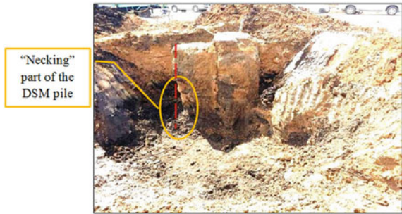
Fig. 10 Trench excavation of trial DSM piles show 'necking' phenomenon
