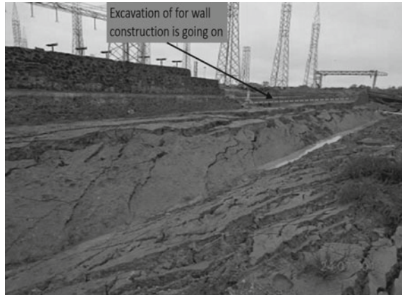
Fig. 4 Collapsed area of buried pipe apx 150 m of pipe along wall was collapsed
