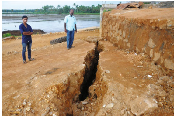
Fig. 4 Failure photographs of Gramenchira Bridge Embankment
