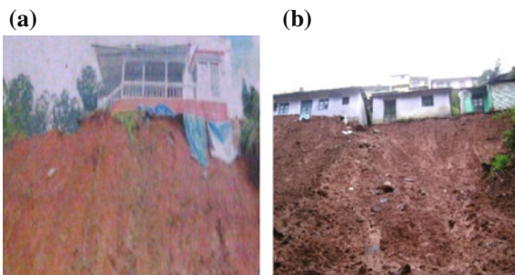
Fig. 5 View of slope failure due to loading the slope at crest; a Kothagiri b Nondimedu
