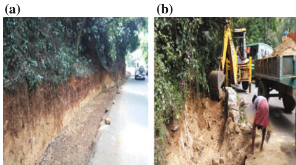
Fig. 3 View of excavation of slope at toe; a and b along Mettupalayam–Coonoor road network
