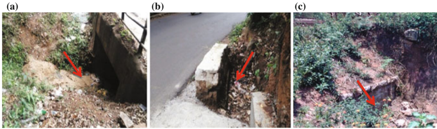
Fig. 6 View of blocking of surface drainage pipe and drainage culvert; a and b along Mettupalayam–Coonoor road network c Aravankadu location
