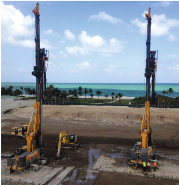
Fig. 11 Hayward Baker’s DAQ system was employed on a job in Miami, USA, for the construction of a sealing slab close to the beach, with stringent positional tolerances
