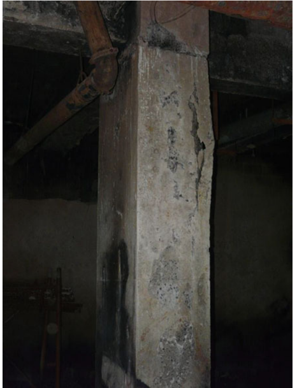
Fig. 8 Spalling of concrete in column along grid 2A1-6 in basement 1 floor
