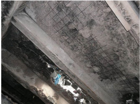
Fig. 7 Spalling of concrete and broken ramp slab with exposed reinforcement—view from basement 1 floor
