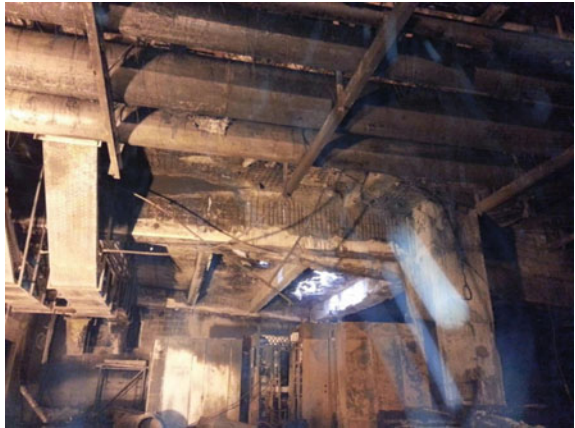
Fig. 9 Spalling of concrete in beam supporting ramp slab in basement 1 floor
