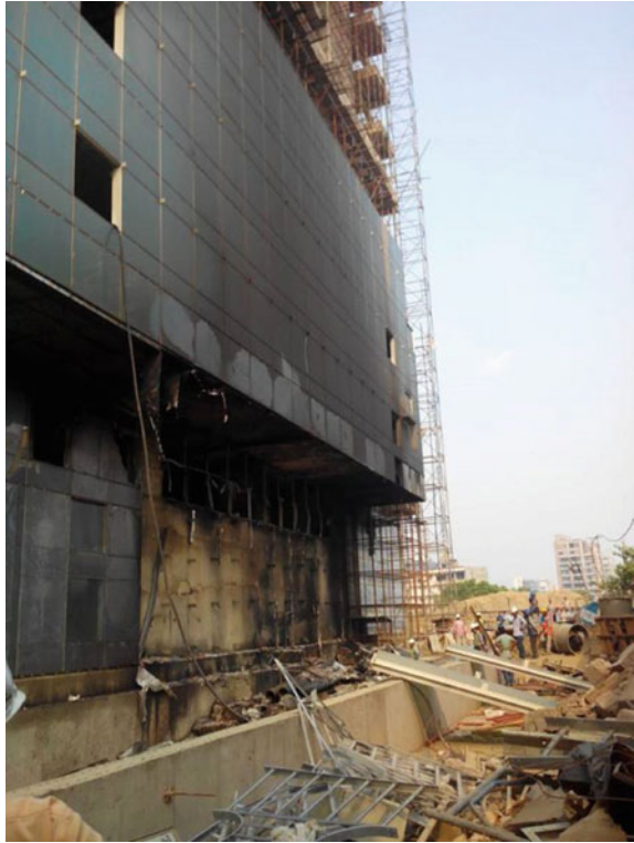
Fig. 4 Fire broke out in basement 1 floor, it got damaged and it passed through the ramp opening and affected the first floor slab and soffit of the second floor slab (there is 4 m cantilever in second floor slab)
