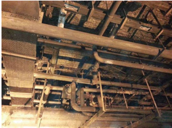
Fig. 5 Spalling of concrete with exposed bottom steel with service lines
