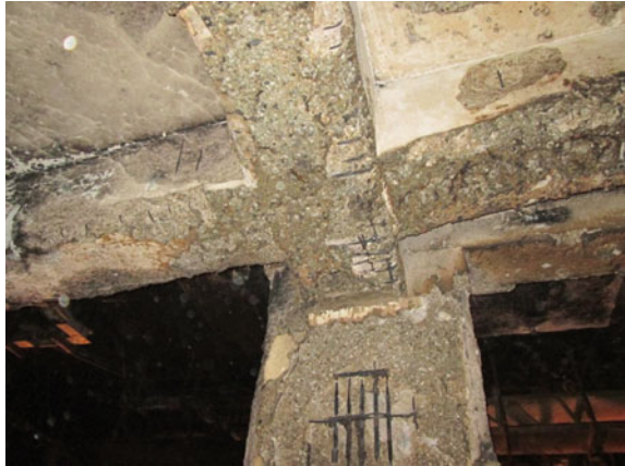
Fig. 10 Closer view of column and beam showing spalling of concrete
