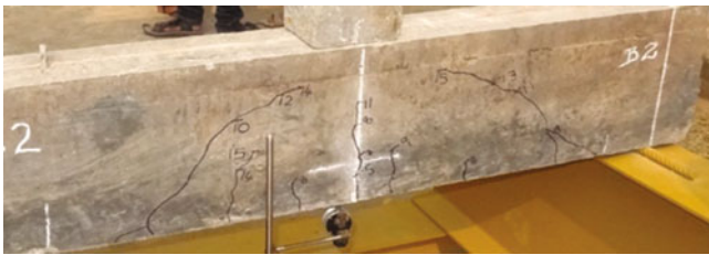
Fig. 4 Failure pattern of B2
