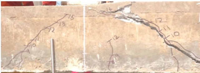
Fig. 5 Failure pattern of B3
