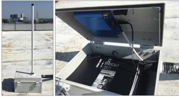
Fig. 3. A gateway is built with LoRa module, antenna, enclosure
