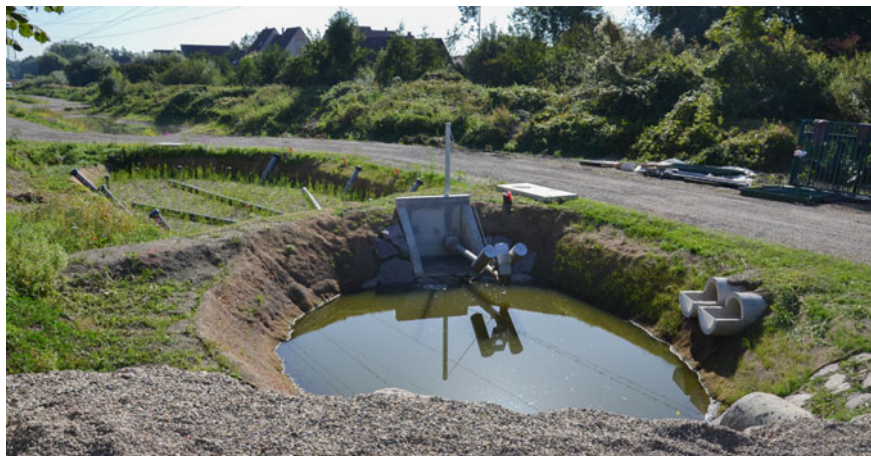
Fig. 4 Hybrid treatment system just after construction. The settling pond is on the lower side of the picture; the constructed treatment wetland is on the upper left side of the picture. A bit further behind, a discharge pond can be seen ( Source ICube Laboratory)
