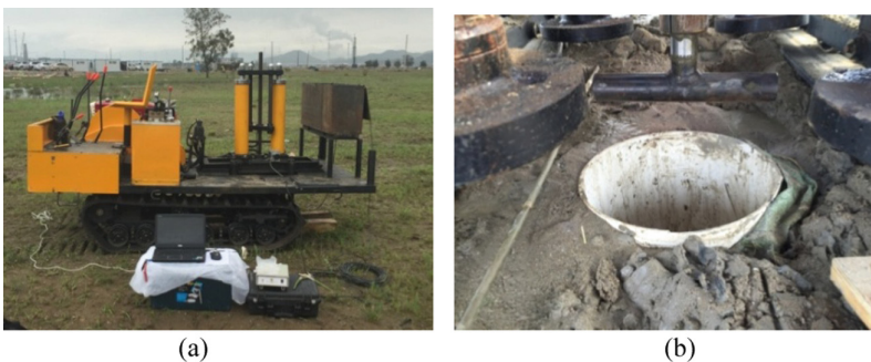
Fig. 5. (a) Equipments, (b) Pre-embedded pipe
