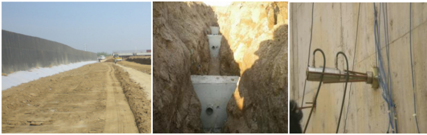
(a) Filling embankment (b) Excavating trench and casting anchor plate (c) Tensioning cables
