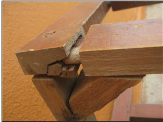
Fig. 3 Broken at the mortise
