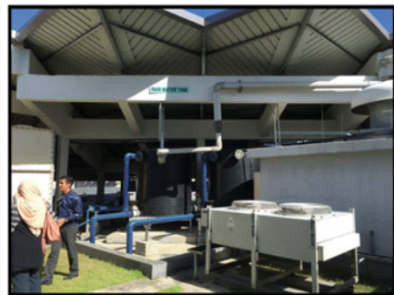
(a) Rainwater Harvesting System
