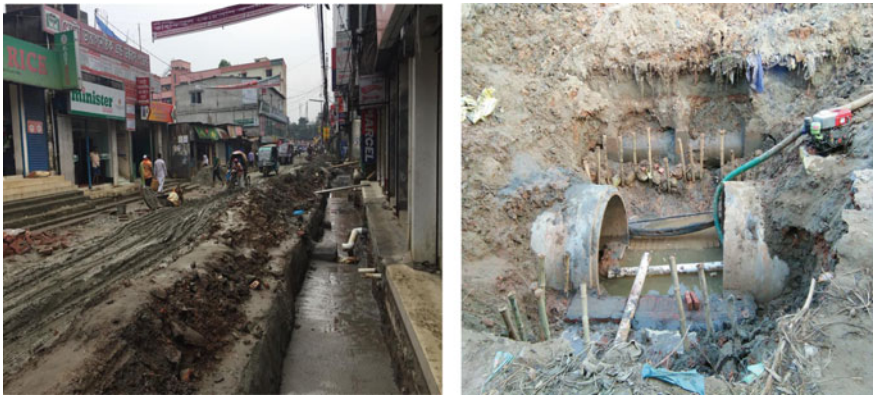
Fig. 8.5 Poor drainage system in Dhaka city. Source Authors
