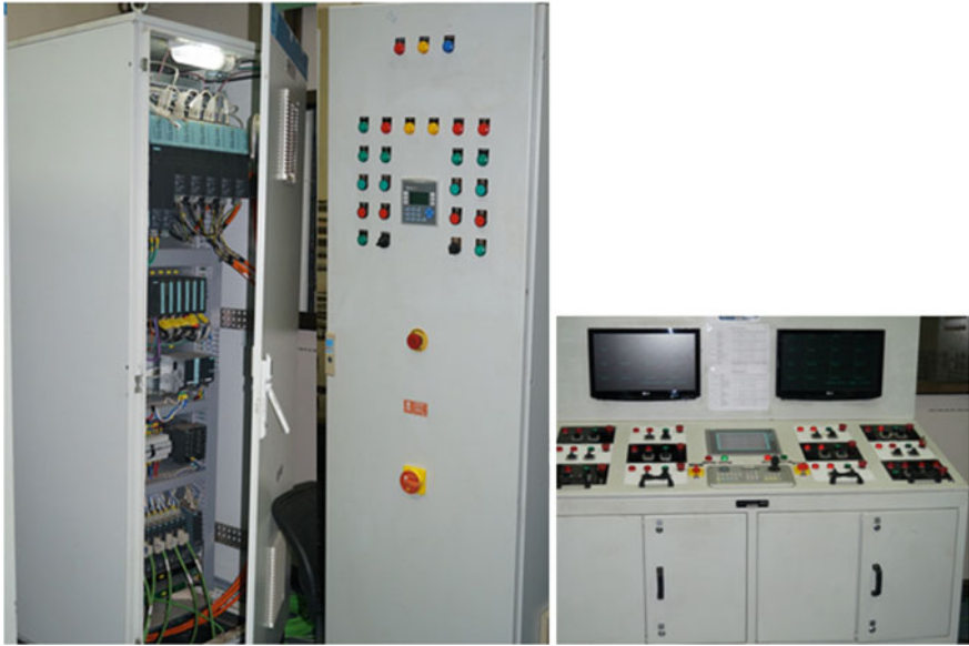
Fig. 10 TDS control panels
