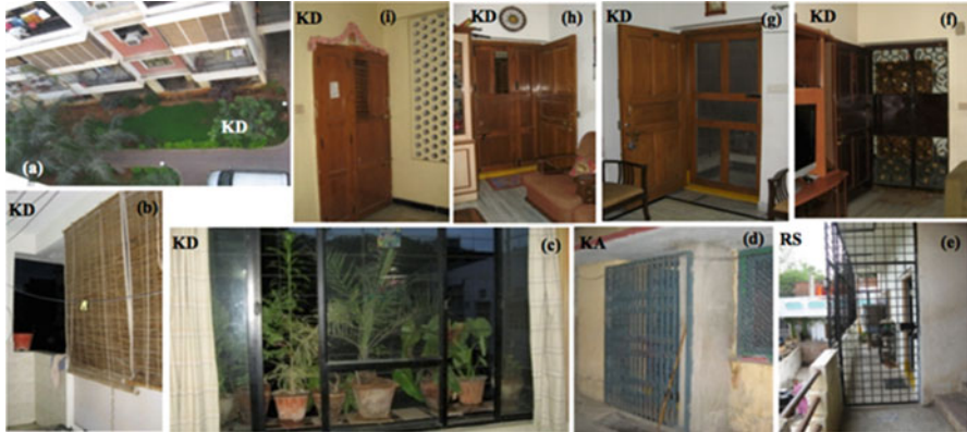
Fig. 25.7 Some interventions applied to windows, doors, and balconies to enhance adaptive operation in Indian apartments (a, b): bamboo blinds hung on balcony openings and (c) planter box extension to windows to reduce glare and sunlight and curtains to improve privacy, (d, e, f) metal grill gates to main doors and metal grill enclosures to balconies to improve safety, privacy, and cross ventilation, (g, h) additional door shutters with mosquito screens and vents for improved cross ventilation, (i) RCC Jalis (grills) applied to corridors for safety, sun control, and cross ventilation [2]
