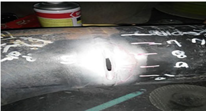
Fig. 11 Pipeline showing crack with measurement
