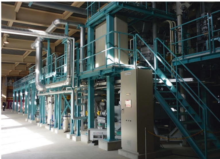
Fig. 9.2 Full-scale plant for P recovery from SSA at the North WWTP of Gifu City
