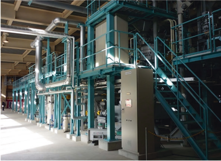
Fig. 9.2 Full-scale plant for P recovery from SSA at the North WWTP of Gifu City
