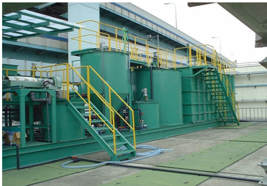
Fig. 35.6 The pilot-scale test plant which was built at the Higashi-nada WWTP in Kobe
