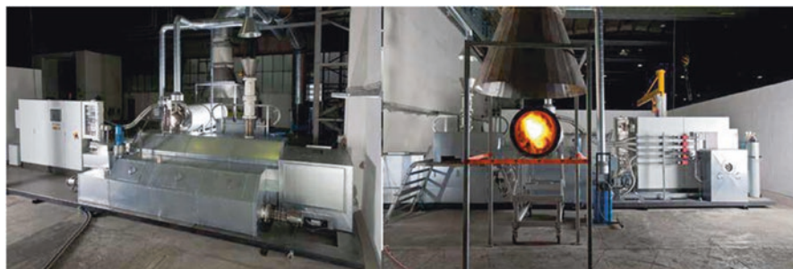
Fig. 29.1 EREKA bioreactor installed in Schwerin, Germany (Hagemann and Kebelmann 2017)
