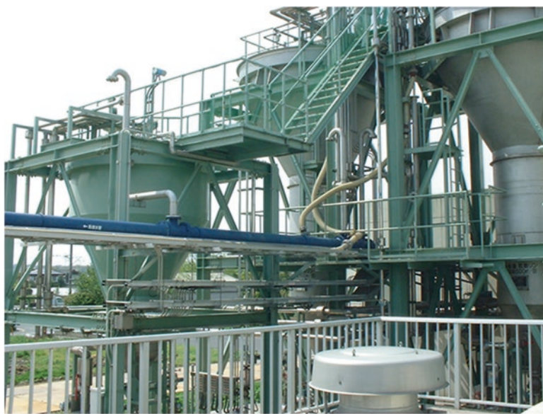
Fig. 1.4 Full-scale plant for recovering struvite from rejected water from a membrane-type solid-liquid separator for digested sludge at Matsue WWTP
