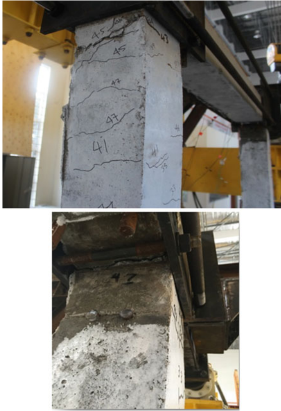
Fig. 31 Crack propagation in the RC bare frame column and connection zone
