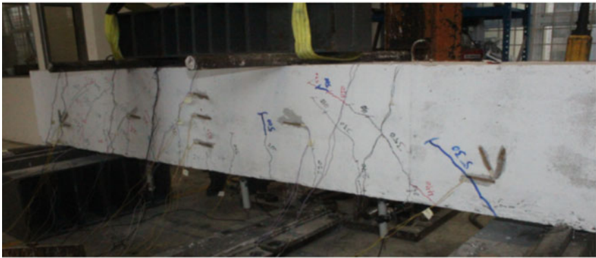
(b) RC crack right view
