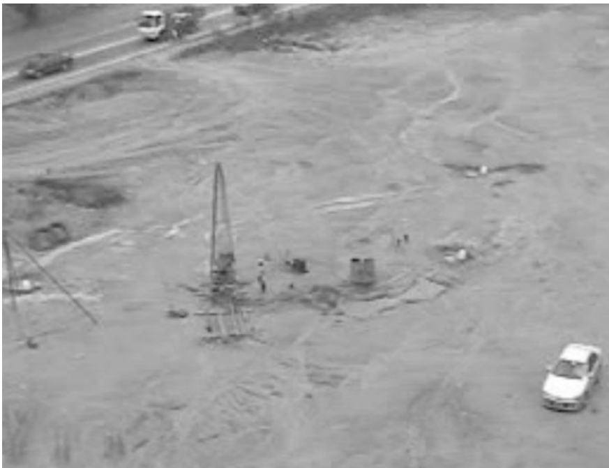
Fig. 3 The samples taken from a borehole drilled on a flat land in Rawang
