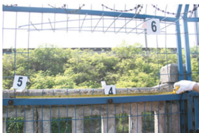
(a) Destroy the metal fence
