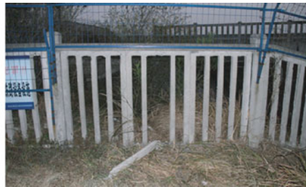
(b) Destroy the cement fence
