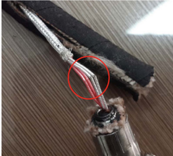
Fig. 5 Damaged part of the extremity of an axlebox temperature sensor
