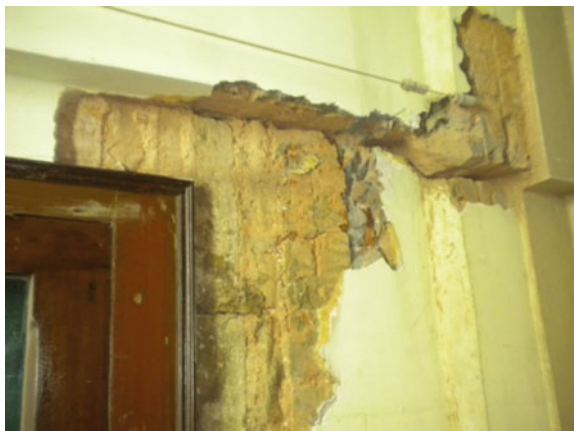
Fig. 2 Damage seen on the wall
