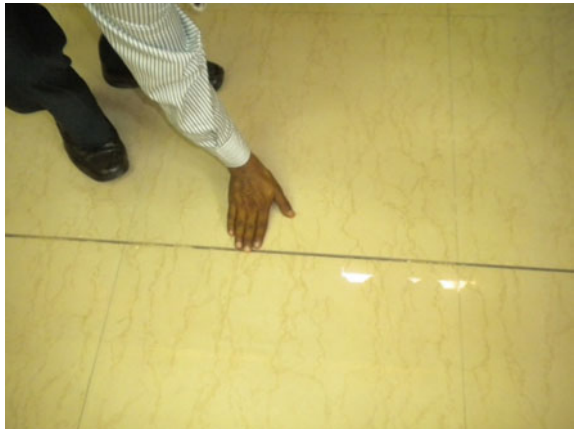
Fig. 4 Differential settlement in floor
