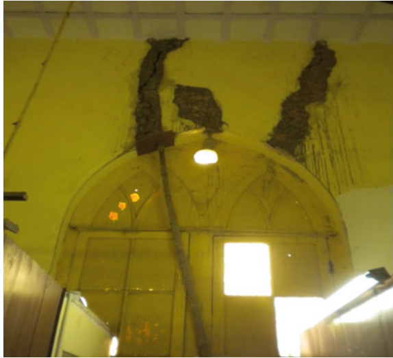
Fig. 3 Distinct cracks seen on wall (N–W) side
