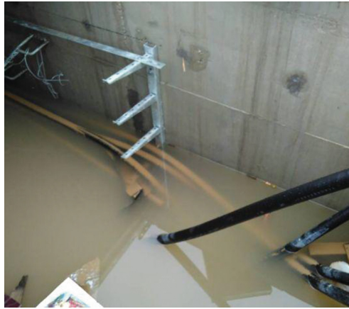
Fig. 1. Cable under spray and immersion accident
