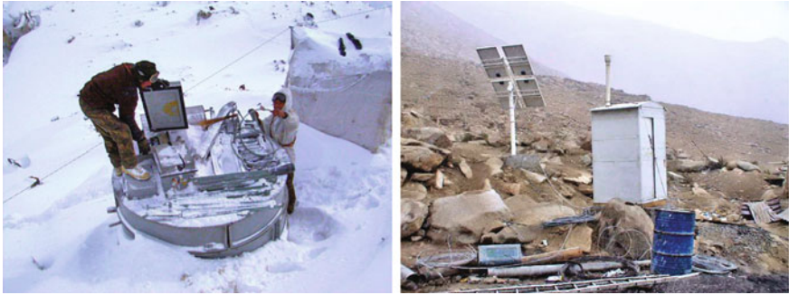
Fig. 3 Temperature-controlled biodigester with toilet superstructure installed at snowbound location in Himalayan region of India. Source Singh and Kamboj (2018)
