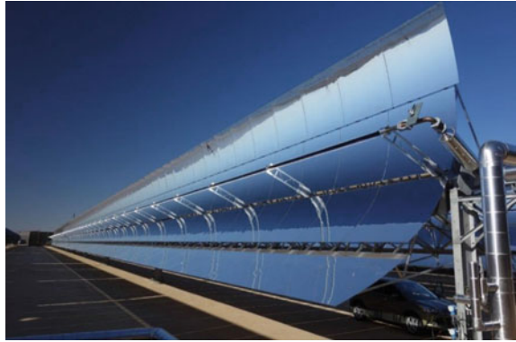
Fig. 4 Installed parabolic trough collector. Image Courtesy: German Flabeg FE GmbH, Flabeg Research and Development Division
