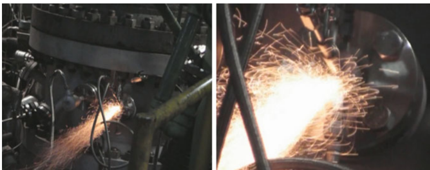
Fig. 4 Syngas flame caused by leakage at the feed nozzle area of the coal gasification pilot plant. (Left) flame at the side-feeding nozzle, (right) enlarged picture on the nozzle area
