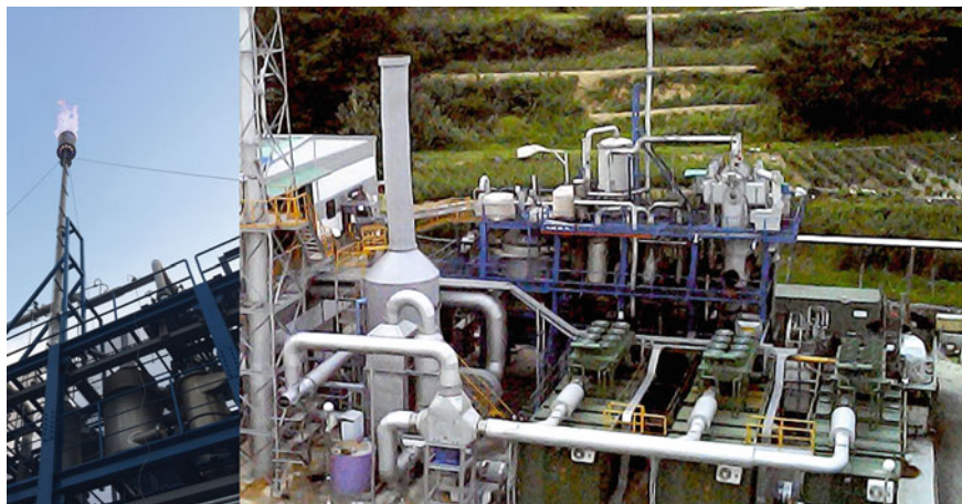
Fig. 3 1 MWh RDF Beltran gasifier system in Korea showing the color of the flame at the flare stack during the commissioning operation
