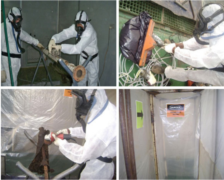
Fig. 5 PPEs used by the allocated trained and licensed asbestos removers and sealed ACM before dismantling
