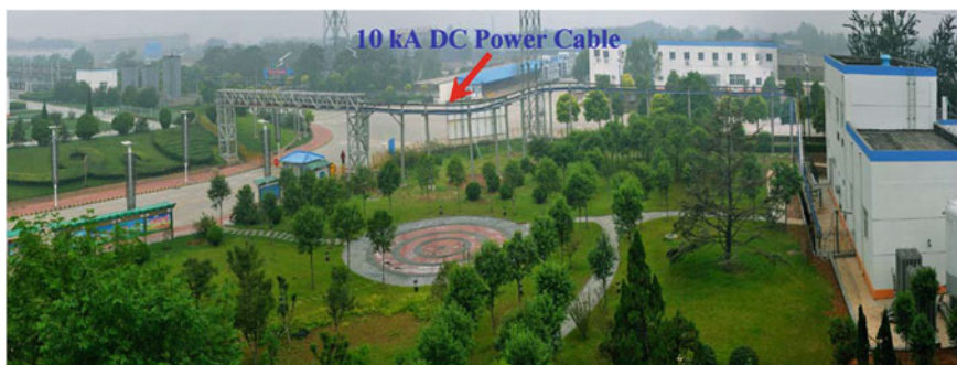
Fig. 3.27 10 kA HTS DC power cable and system in Henan, China
