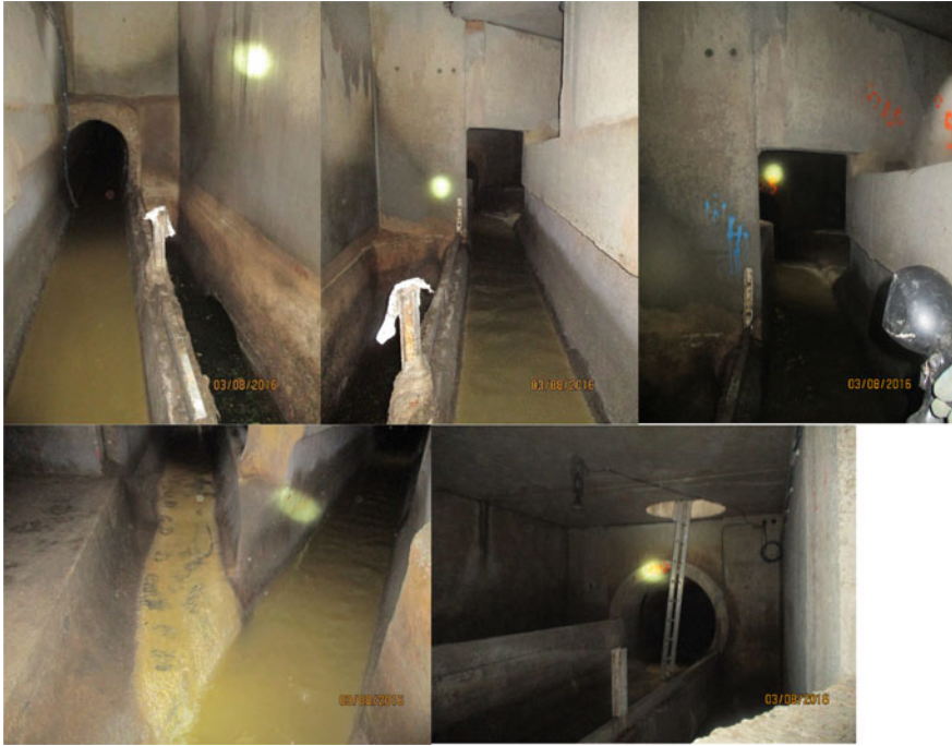
Fig. 5 Pictures of a visit to a stormwater regulator—Haguenau (France)
