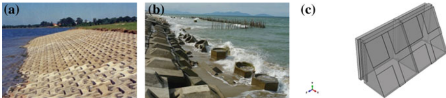
Fig. 3 a Inter-locking blocks forming RS structure, b RS structure failure, and c illustration of thin-wall RS structure from BUSADCO, Internet
