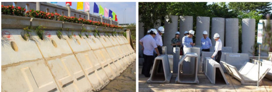
Fig. 1 Several blocks shape have been built to protect coast and riverbank (Source http://busadco.com.vn/en/ )
