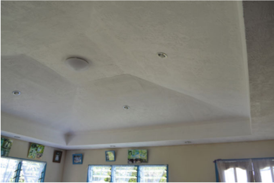
Fig. 26.4 Raised vaulted ceiling of the loto fale owned by the 'Āliki family. Note the textured surface created by paint-dipped plastic bags shaped into flowers that designates this space for 'display' and hospitality ( Photograph Charmaine 'Ilaiū Talei)
