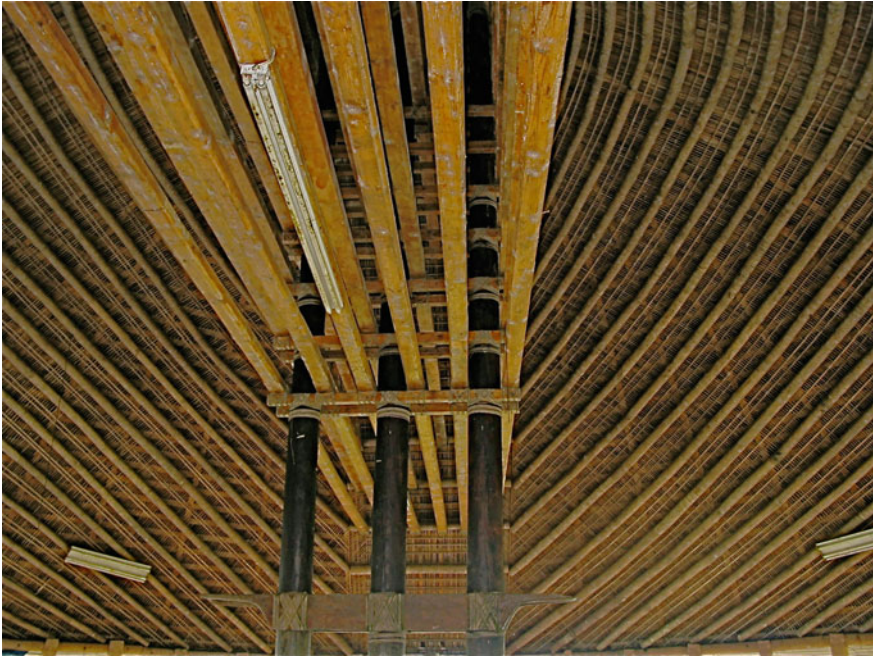
Fig. 24.3 Interior view of the roof of a fale tele with three central posts, Leone, Tutuila and American Sāmoa (Photograph Micah Van der Ryn)
