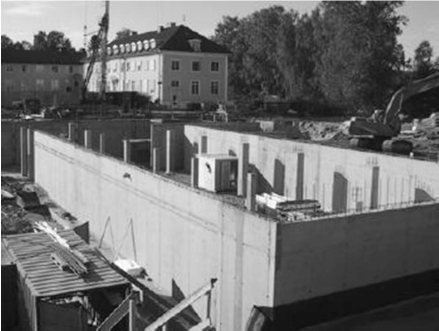
Fig. 1.8 New high school building in Norway (Mehus and Hauck 2002), in which 35% recycled coarse aggregates were used in foundations, basement walls, and columns
