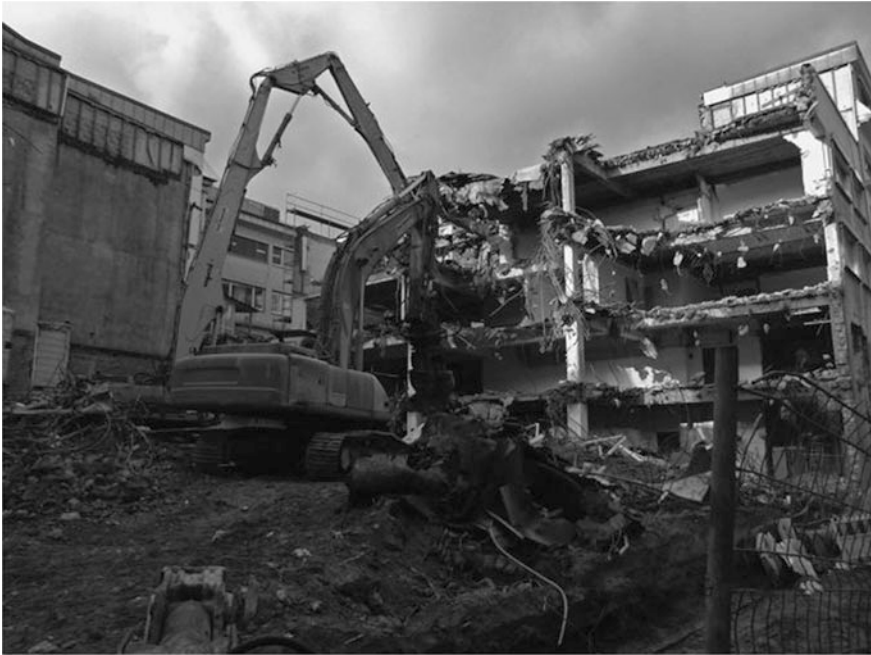
Fig. 2.6 Typical demolition from top to down. After demolition of all non-bearing structures, the bearing columns are left. In the next step, the columns will be demolished beginning with the top level. After that the demolition starts again with the next field (Kamrath 2013 )
