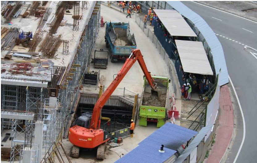
Fig. 7. Long-arm excavator was removing spoil material through opening within the ground floor slab
