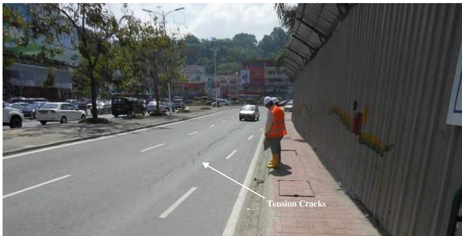
Fig. 11. Ground deformation and cracks on the road pavement
