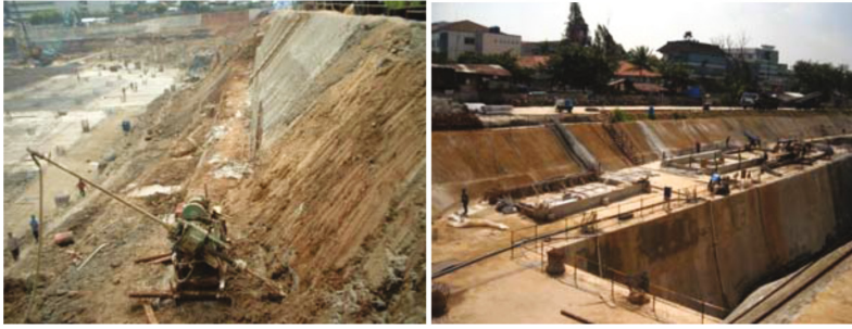
Fig. 8. Excavation with combined soil nailing at upper slope and steep cut for excavation at south of Jakarta
