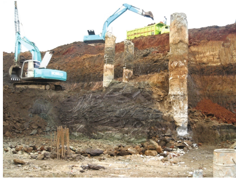
Fig. 10. Strong layers of soils alternating with the cemented sands are found at South Jakarta
