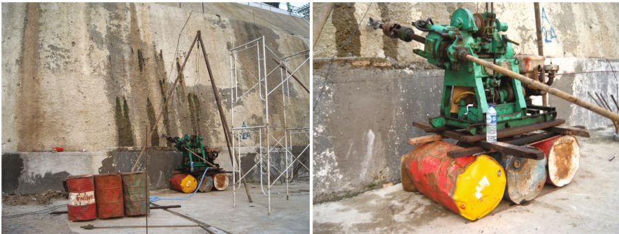
Fig. 9. The use of horizontal drains to drain out ground water seepage for stable slope at South Jakarta
