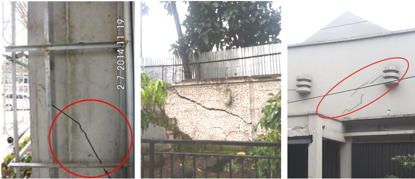
Fig. 21. Typical damages of buildings due to settlement caused by dewatering (Rahardjo 2016)
