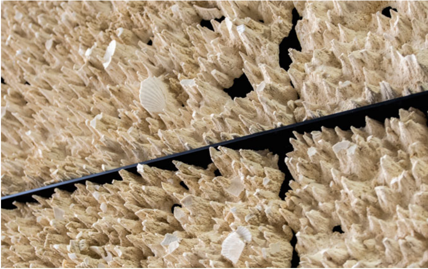
Fig. 8. Detail of limestone wall illustrating topological diversification and material perforation. ©ICD, K. Rinderspacher
