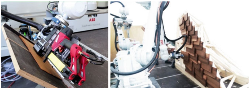
Fig. 8. Left Robotic scanning and gripping. Right Mounting and fixation of timber panel. We used hand-split timber panels of variable widths between 8 and 30 cm and a fixed height of 60 cm
