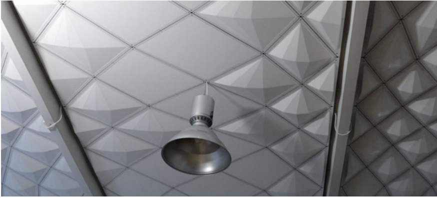
Fig. 10. Realized adapted acoustic ceiling
