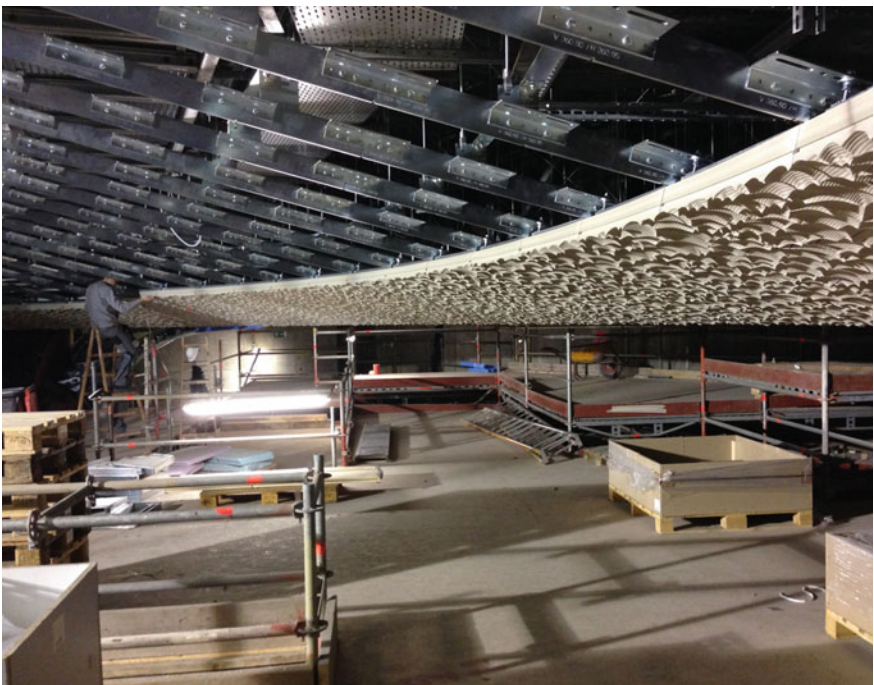
Fig. 8. Ceiling panels being assembled onto the substructure on site. Photo by the author
