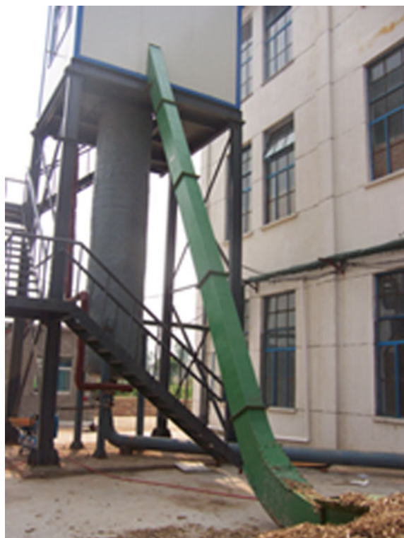
Fig. 8.4 5 m 3 steam explosion tank
