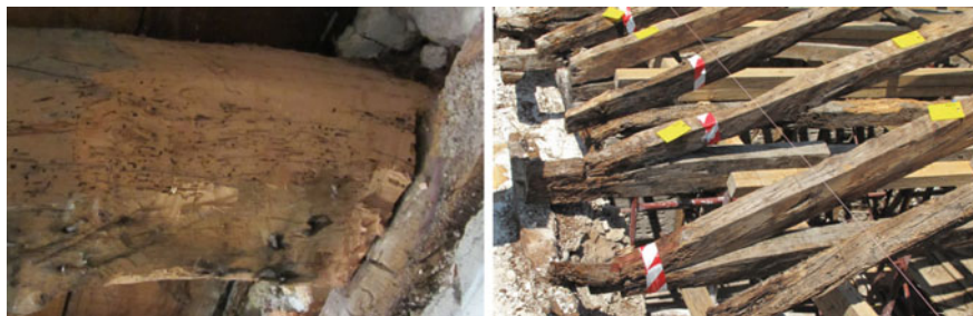
Fig. 25 Examples of decayed old timber end beams that can be found both in floor and roof systems
