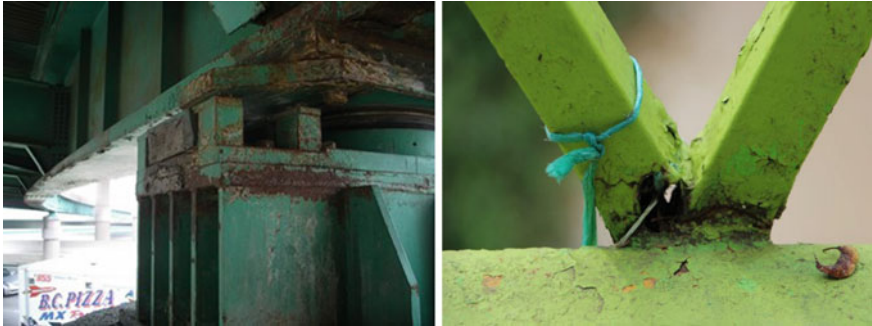
Fig. 17 Corrosion in bridge structural elements
