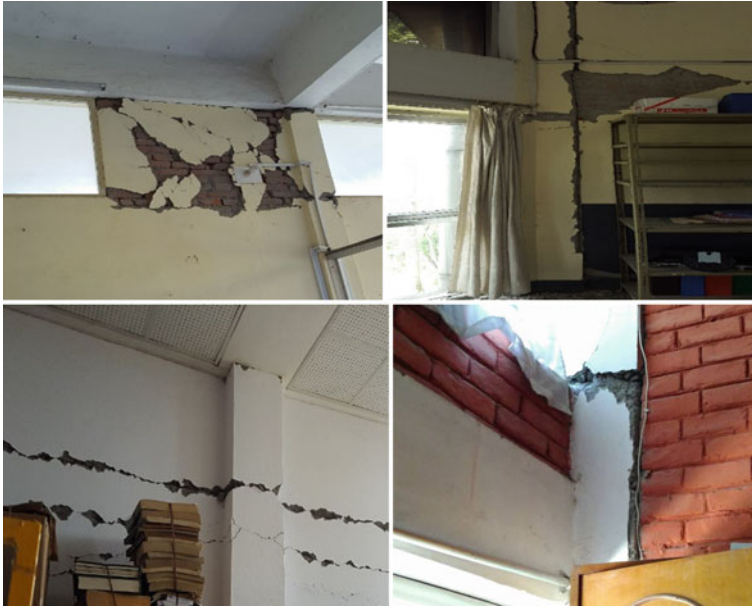
Fig. 6 Damage observed in Kathmandu University Central Library (Dhulikhel) after the major earthquake
