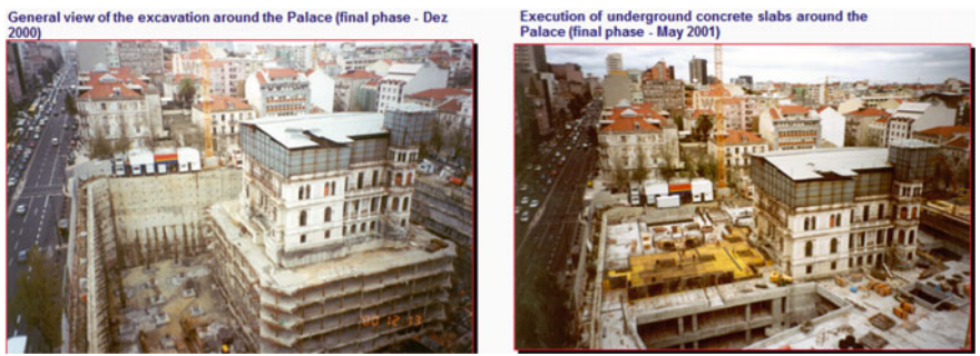
Fig. 18 Final phases of excavation and construction of underground slabs around the palace
