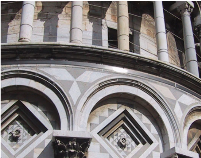
Fig. 4 Leaning Tower of Pisa; Pretensioned circumferential tie realized with a removable stainless steel band
