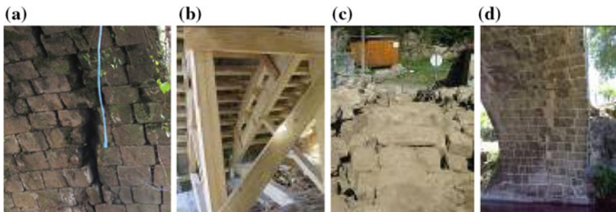
Fig. 9 Esmoriz Bridge: a View of the arch intrados before the intervention, b Falsework, c View of the arch extrados after infill removal and spandrel walls' dismantling, d View of the arch intrados after reconstruction
