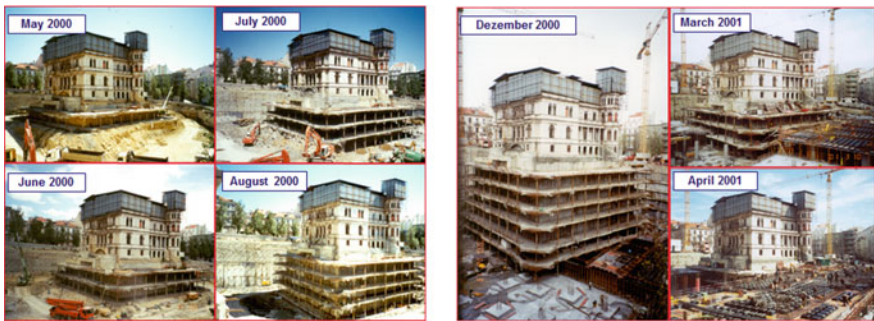
Fig. 16 Sequences of excavation and construction of the underground slabs around the Palace
