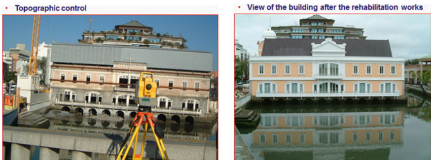
Fig. 23 Topographic control and view of the building at the end of the refurbishment works
