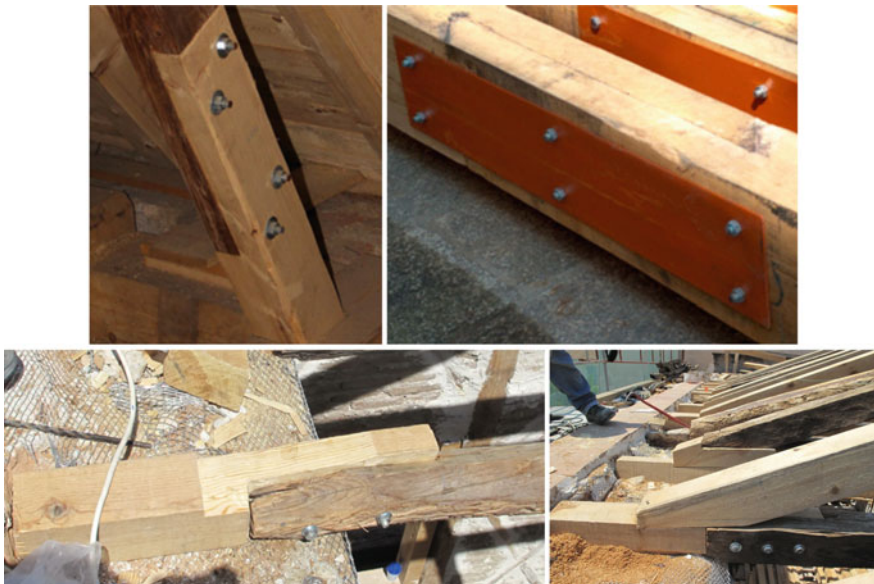
Fig. 12 Scarf joints reinforced with metal fasteners and plates. Prosthesis with scarf joint and bolts realized at the heel joint of a roof
