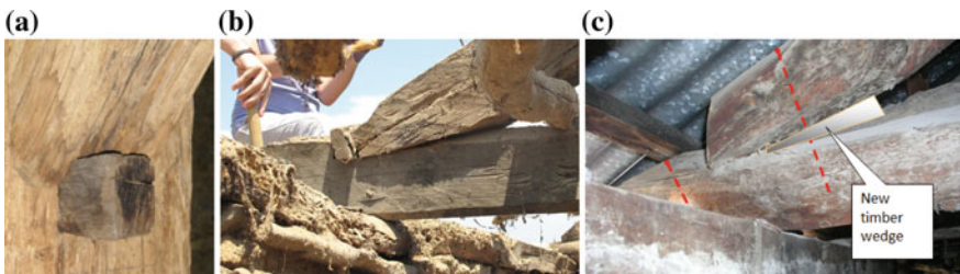
Fig. 3 a Tenon and mortise joint: additional wooden wedge used to ensure a tight contact between the tenon and the mortise, b additional wooden piece to ensure the contact of the timber elements, c proposal for the reinforcement of a poorly constructed heel joint. Addition of a new wedge and screws
