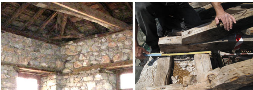
Fig. 30 Roofs nailed on timber ties that connect the vertical load bearing walls of the buildings (masonry or timber-framed) improving their seismic resistance [15, 16]
