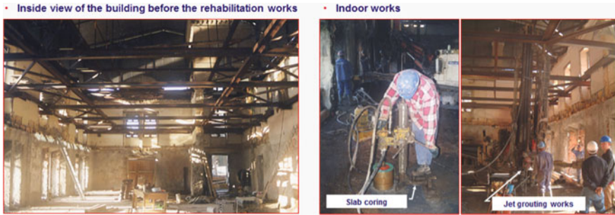
Fig. 20 Inside view of the building before the rehabilitation works and indoor slab
