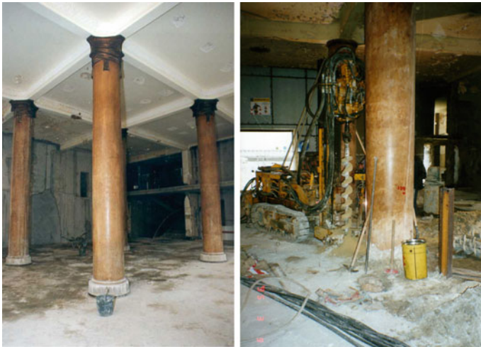
Fig. 8 Rivoli theatre building: Rivoli theatre building: execution of H steel piles (drilled borehole of 0.20 m diameter)
