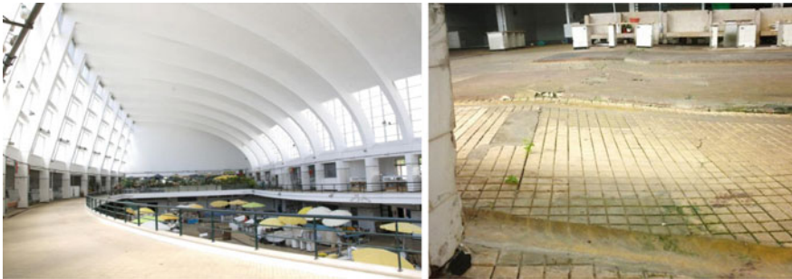
Fig. 24 The building of “Bom Sucesso” market in Porto and settlement of the ground level
