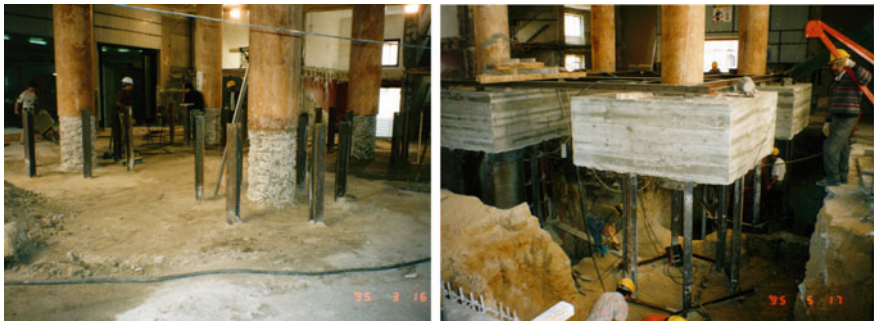
Fig. 10 Rivoli theatre building: preparation of the pillar to connect the reinforced concrete minipiles' cap and the execution of the structure of the pillar suspension, concreting of the definite pillar with the bracing reinforcement
