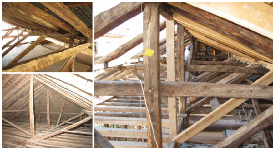
Fig. 21 Post and beam type of roofs of Post-Byzantine mansions in Greece [14, 16]. Excessive deformation of the longitudinal horizontal beams that support the rafters. Reinforcement by adding just new timber struts
