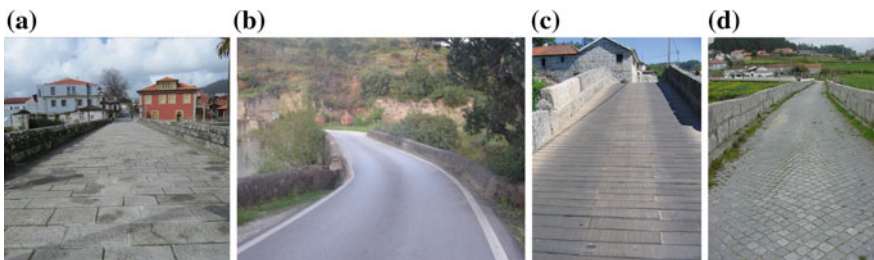
Fig. 7 Pavement repair: a Replacement of masonry stones, b Bituminous pavement overlay and c, d Replacement pavement
