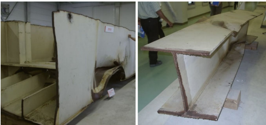
Fig. 18 Damage to structural elements caused by the 1995 Kobe earthquake
