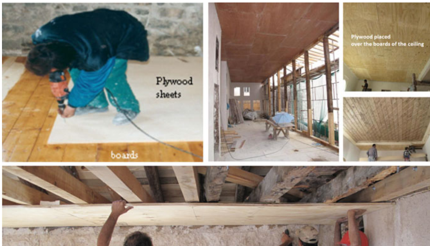
Fig. 31 Use of plywood panels over the existing floor boards and under the second layer of boards for the pavement. Use of plywood panels between the horizontal tie-beams of the roof and the boards of the ceiling for the improvement of the diaphragmatic action of the floor and the roof
