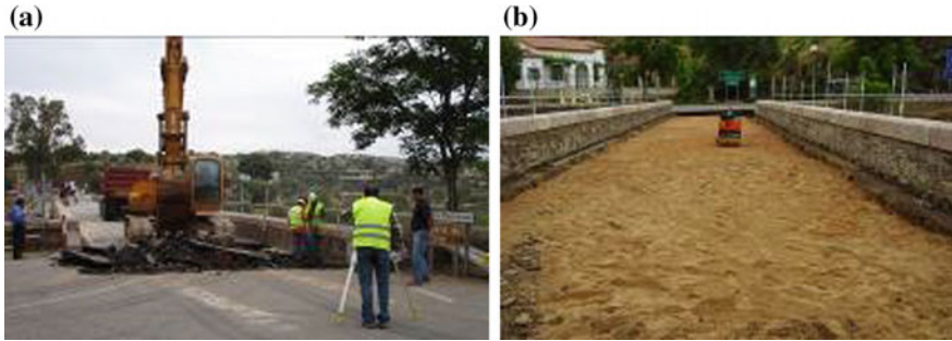
Fig. 13 Segura bridge: a Bituminous removal and b Surface regularization for the application of a concrete slab on the pavement [21]
