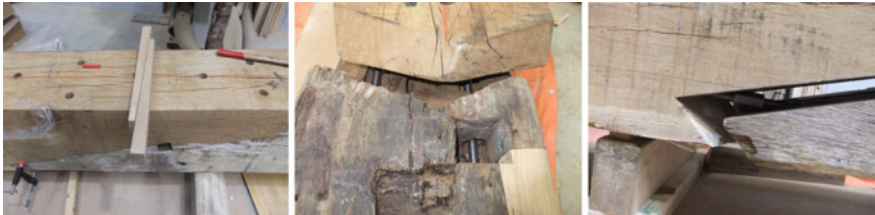
Fig. 14 Scarf joint reinforced with glued in rods: steel rods are glued in both timber members and connected with a long nut. Credits Pascal Lemlyn. Restauration du Moulin de l'abbaye de la Paix Dieu, Institut du patrimoine Wallon, Belgique
