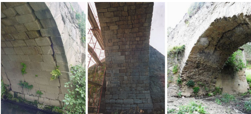
Fig. 2 Longitudinal cracks due to the bridge structural performance in the transverse direction
