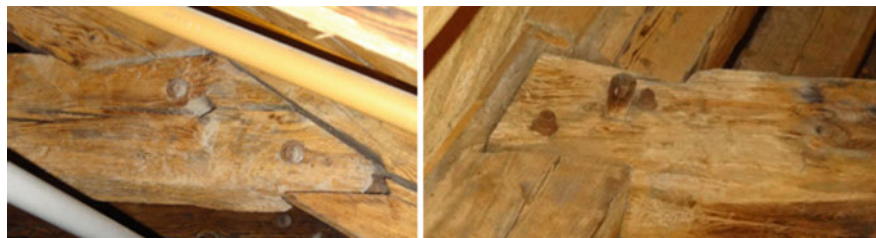
Fig. 11 Traditional reinforcement of dovetail-lap joints under tension loads by adding wooden dowels
