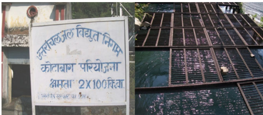
BROKEN COVER SCREEN
