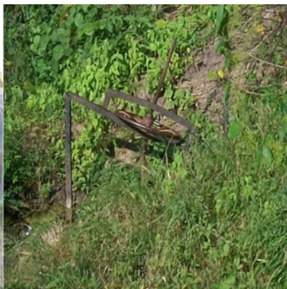
SLUICE GATE WAS BROKEN
