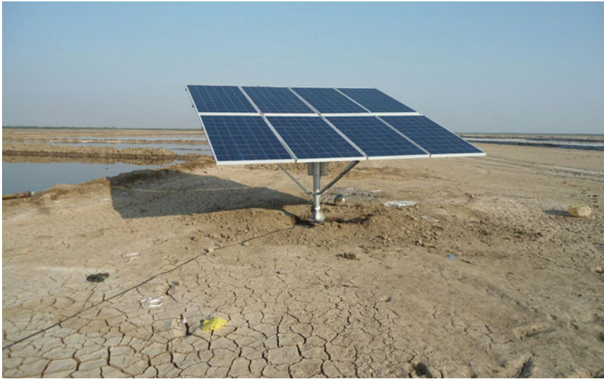
Fig. 1 Solar water pumping system for irrigation
