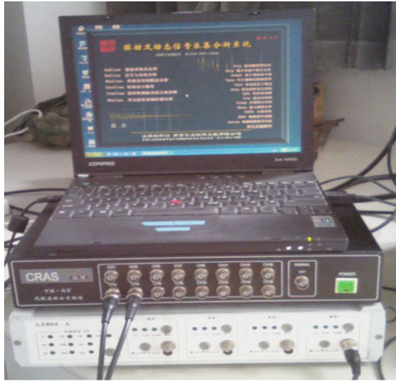
Fig. 7 Signal conditioning and data acquisition instruments
