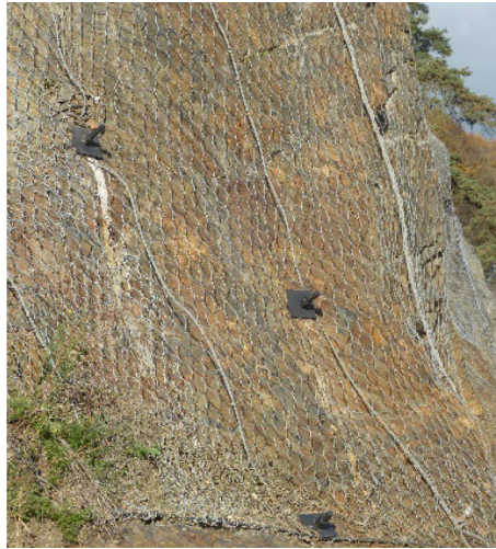
Fig. 1. Anchoring high-strength steel mesh to the bedrock in the Štěchovice area, Czech Republic
