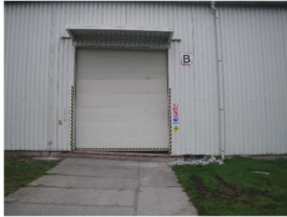
Fig. 4. The consequence of ground descent to the warehouse.
