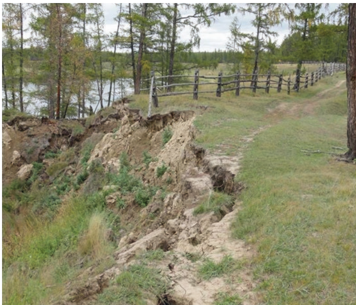
Fig. 11.5 Destruction of roads by thawing of frozen ground. Megino-Kangalasskii ulus (district), Suola village, 2010
