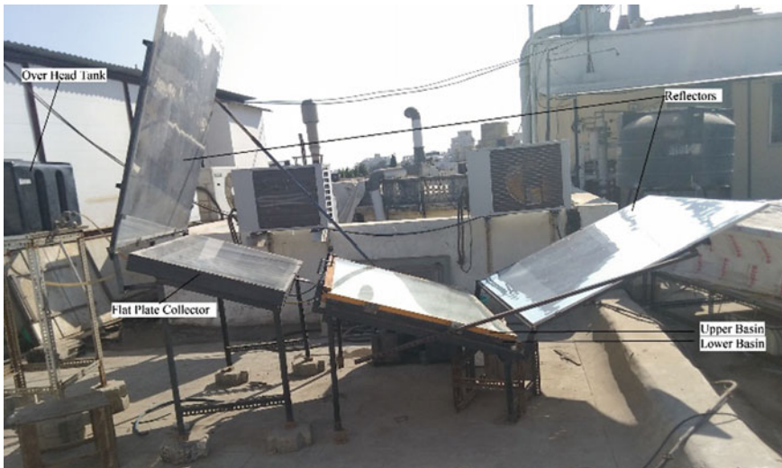
Fig. 2 System at CSIR-CSMCRI, Bhavnagar
