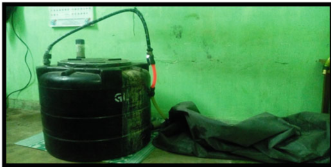
Fig. 2 A 200 l digester and gas collector
