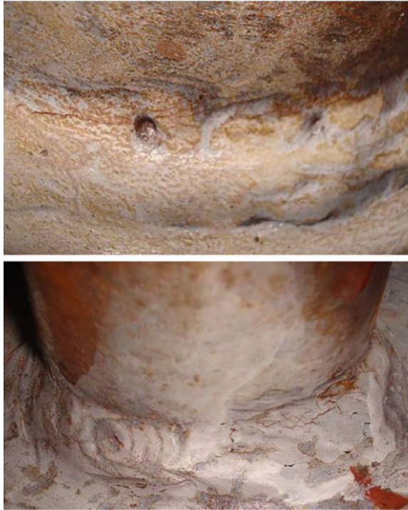
Fig. 1 Defects of fillet weld of boiler tube
