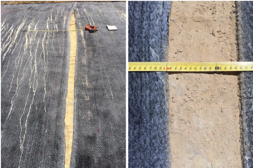
Fig. 23.4 Zone of seam separation and seam gap
