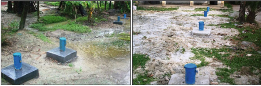
Fig. 26.2 Examples of installed nest of piezometers at Kolapara, Patuakhali (left), and Barisal Sadar (right)
