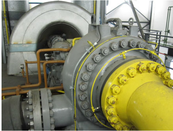
Fig. 5.1 A gas compressor
