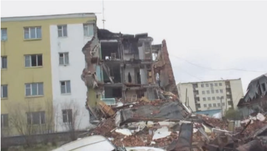
Fig. 22.16 Collapse of the building due to permafrost thawing, photo by V.E. Romanovskiy
