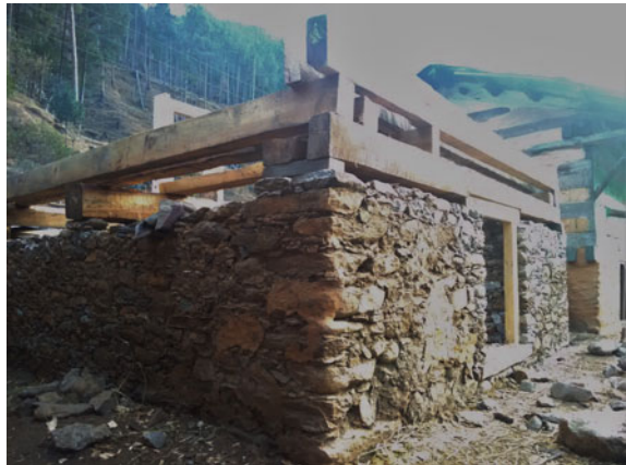
Fig. 9 On-going contemporary construction in typical Koti banal style of architecture in village Purola
